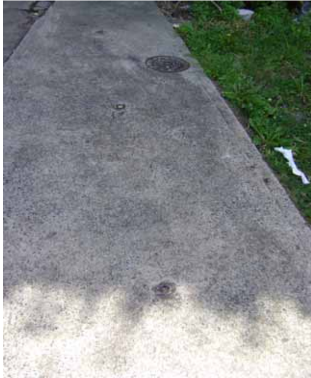
Photo 3 - associated tank infrastructure
