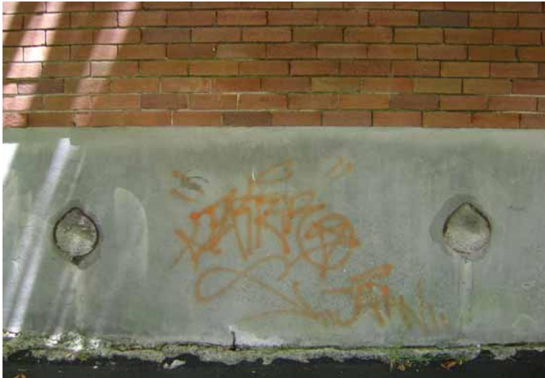
Photo 13 - Fill points on building in Fred Street
